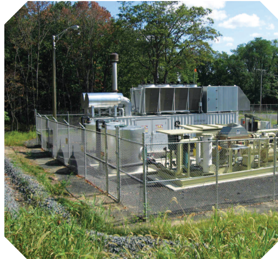
Monmouth County's one megawatt sustainable biopower project produces enough energy to support their materials processing and recovering facility.
